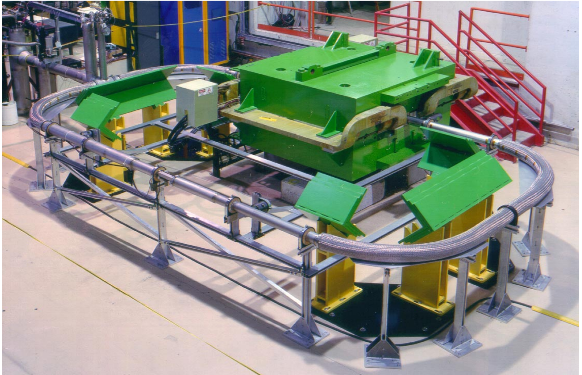
Figure 5. The Fermilab Transmission-Line Test Facility. The conventional magnet is configured as a DC transformer; the secondary is a superconducting loop. This facility has been energized to over 100 kA, and has a four meter long replaceable section used to test various conductor and splice configurations.
